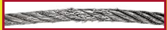
Figure 1: Tightlining as shown in this photo creates extreme pressure on the hoist rope.
