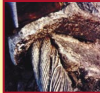
Figure 2: Severely Deteriorated Wedge
